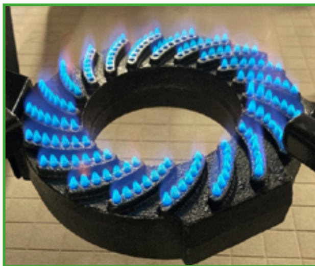
A blue flame, sitting correctly on the burner – an indication that the appliance is correctly ventilated.
