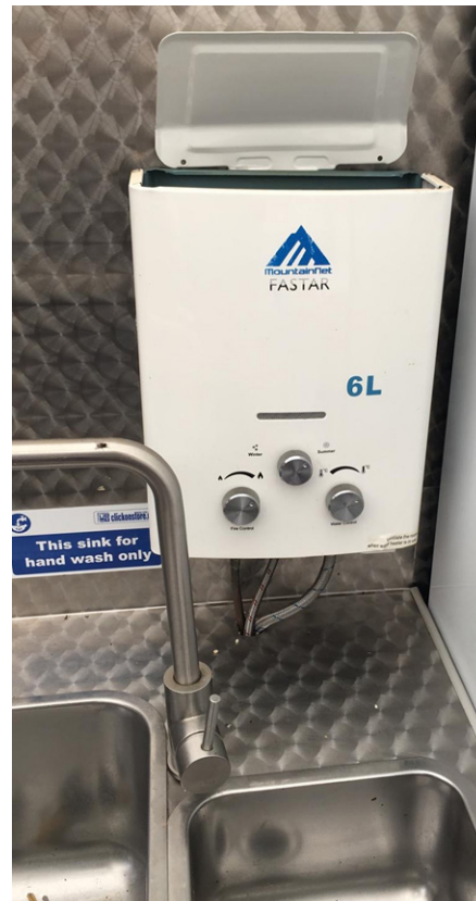
Photo: Example of a water heater
